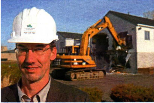
Photograph by Richard Sennott, Star Tribune Building demolition, for expansion at West Lutheran High School
